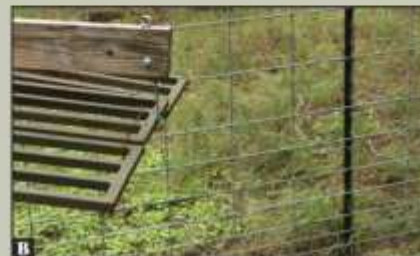
Once in place, the hook and eye latch set holds the panels up (B).
